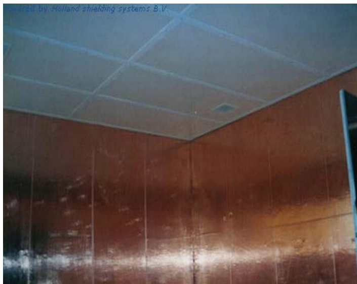
Screened dismountable ceiling
